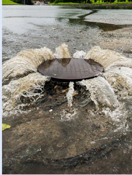
Overbelastet kloaksystem under skybrud
